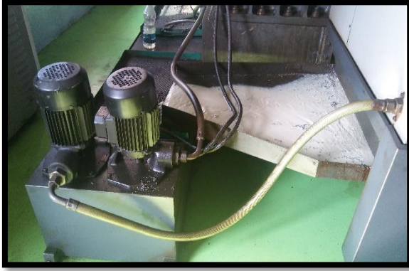
Figure 13: Reduced leakage of coolant
