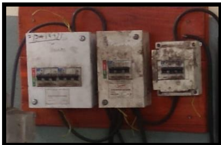
Figure 2: Improper wire junction
