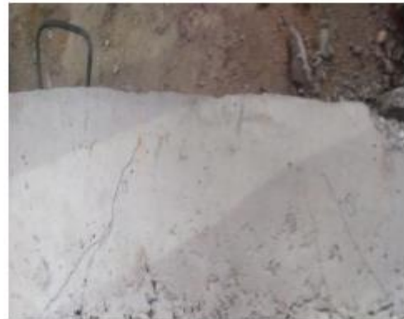
Fig. 13. Initial cracking in BL1 beam
