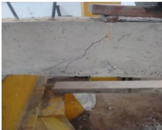
Fig. 12. Cracking pattern in BR1 beam
